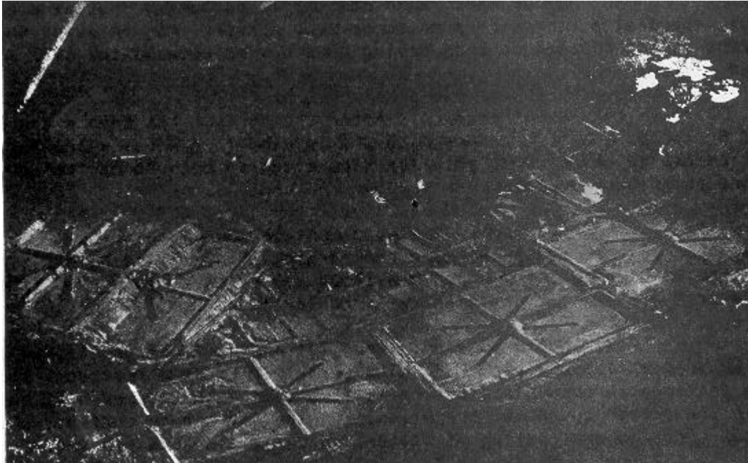
Figure 2-17. Aerial view of wastewater treatment plant with intermittent sand filters. (In each set of four beds, distribution troughs for dosing radiate from a central diversion box.)
